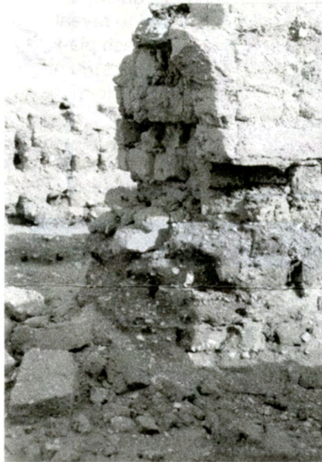
North Palace wall showing the deterioration before re-construction
